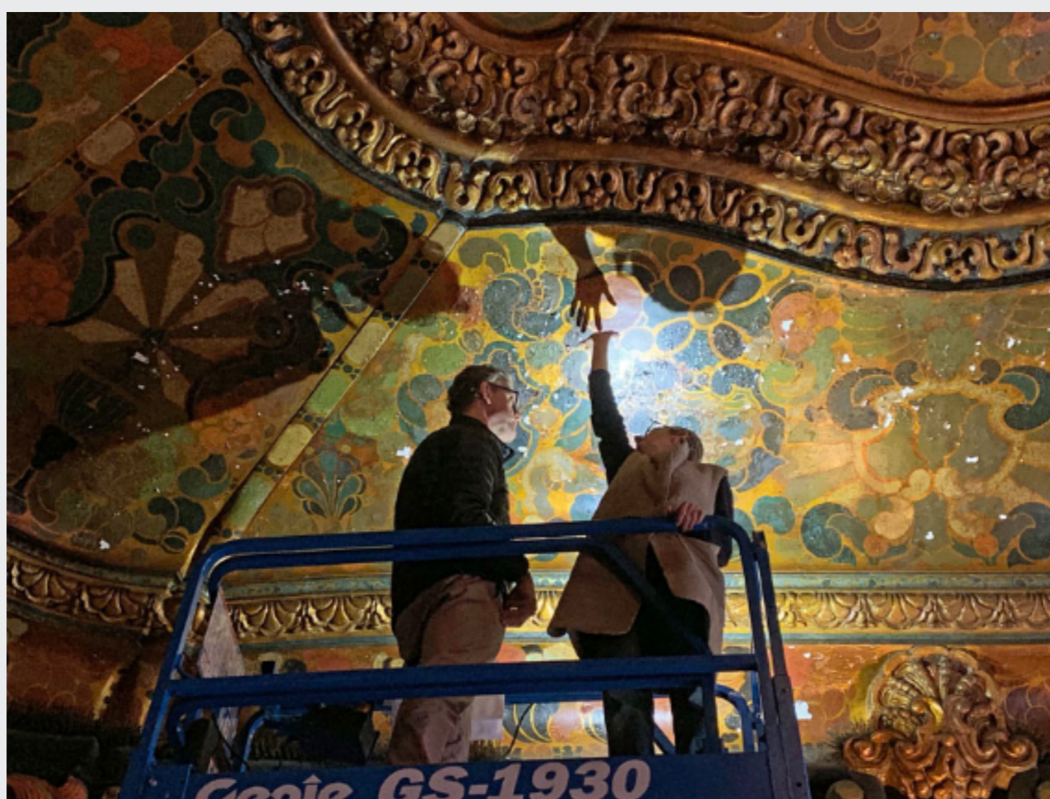
Assessing gilded and stenciled surface finishes of the ticket lobby (© Building Conservation Associates Inc)
