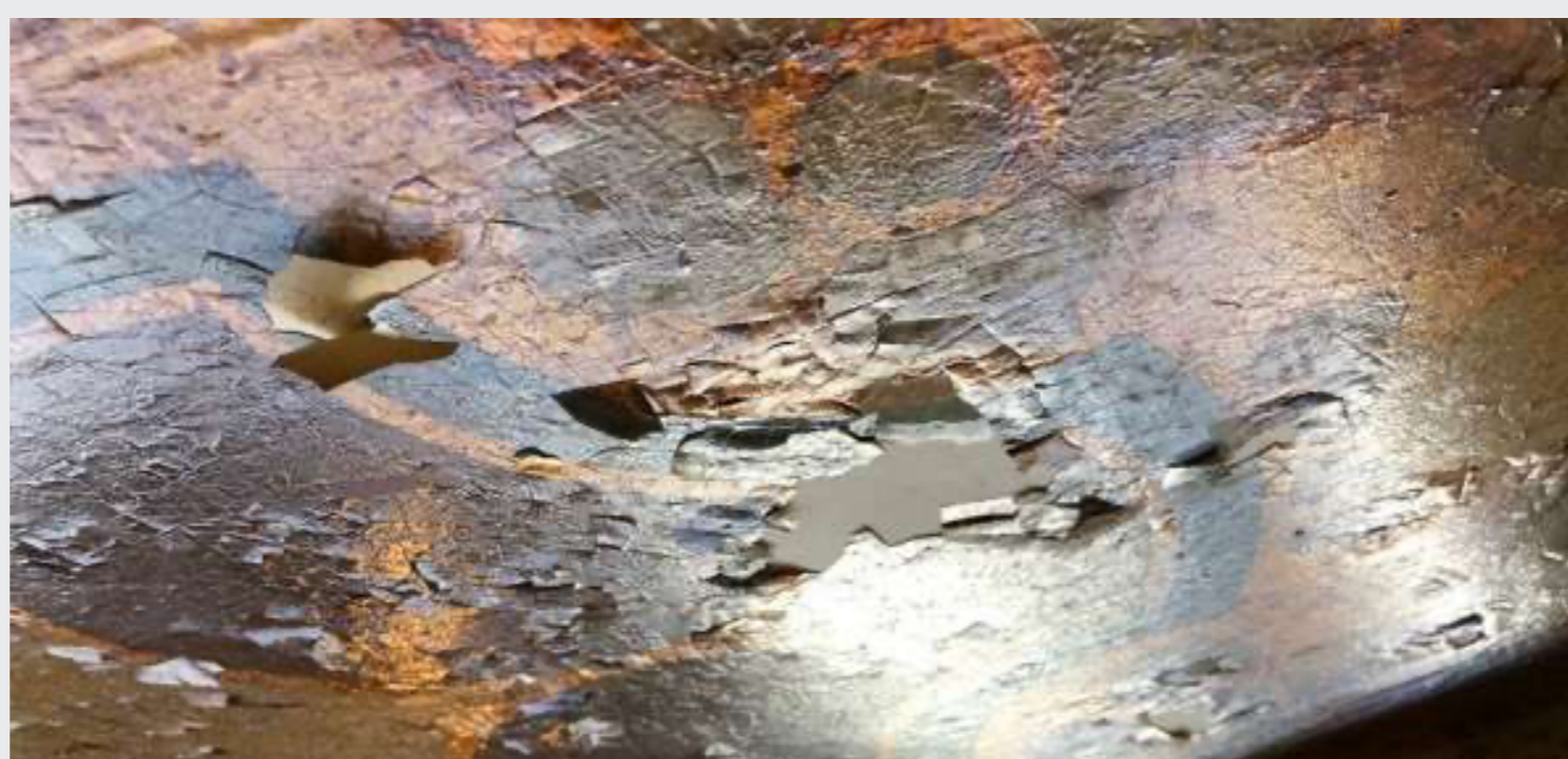
Closeup of painted surfaces exhibiting lifting finishes (© Building Conservation Associates Inc)
